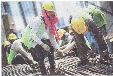
Accidents caused by poor safety management at construction sites are serious and must be addressed.
